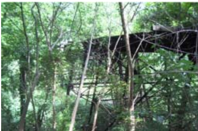
Foundry Branch Trolley Trestle: Crossing Foundry Branch in Glover Archibald Park. (DCPL Archives)
